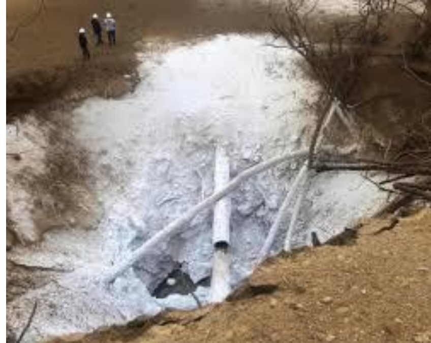
Site of carbon dioxide pipeline rupture in Satartia, MS in February 2020. Credit: Yazoo County Emergency Management Agency
